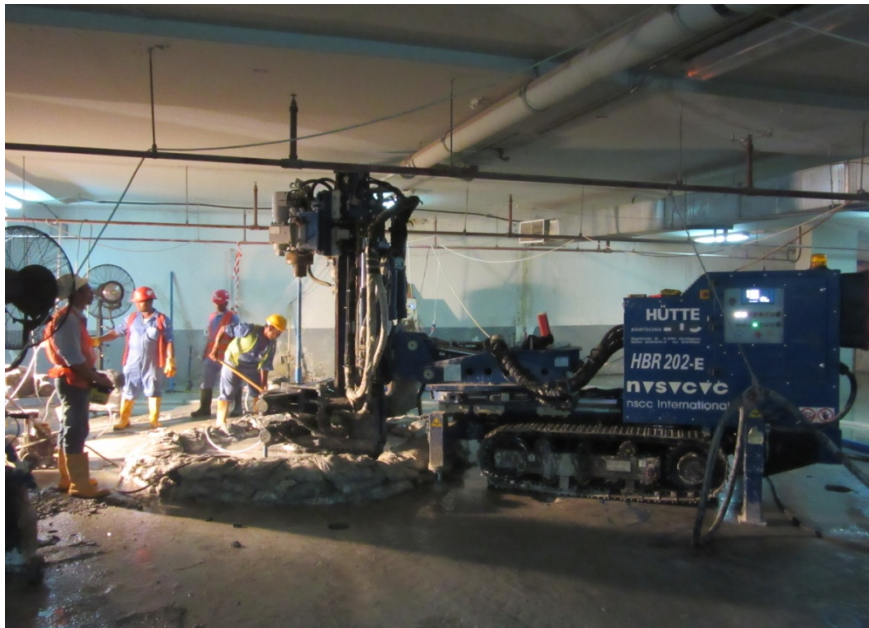
Figure 10 – Electric Drilling Rig
